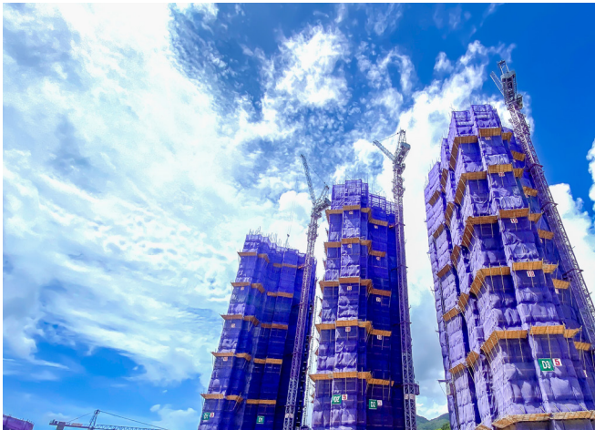
Installing anti-collision systems and deploying 5G-enabled unmanned tower cranes at our Sai Sha Development Project
