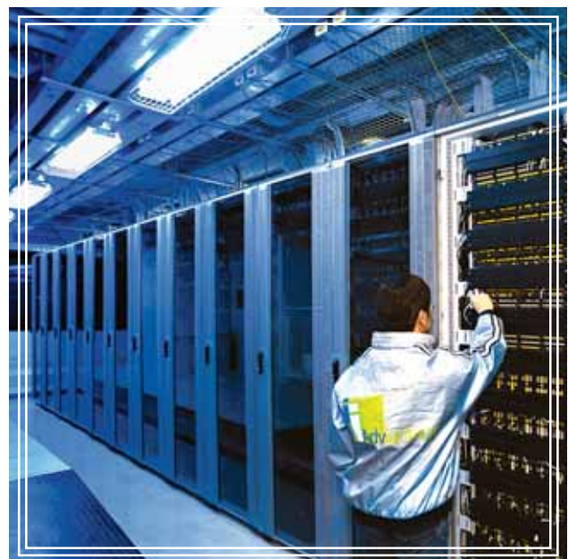
SUNeVision's iAdvantage provides world-class data centre facilities and service
